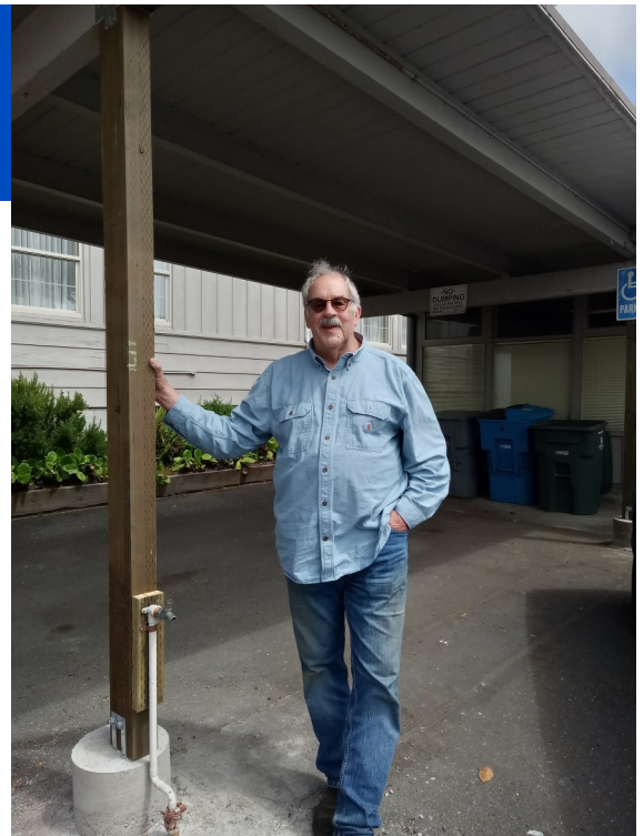
Jim showing off the new sturdy supporting posts for the carport roof which has become the handicapped parking space.
